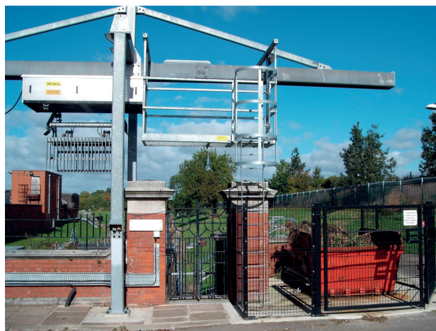
Bosker trash rake installation at Thames Water's Walton-on-Thames water treatment works
