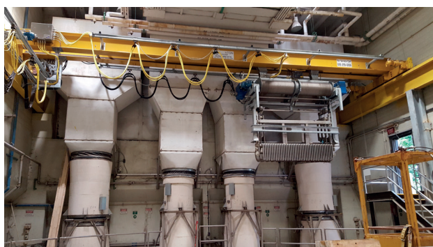
Bosker deep raking system installed on a 110-metre-deep inlet screen
