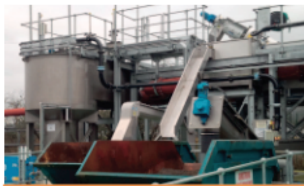
Jacopa-jeta grit removal plant
